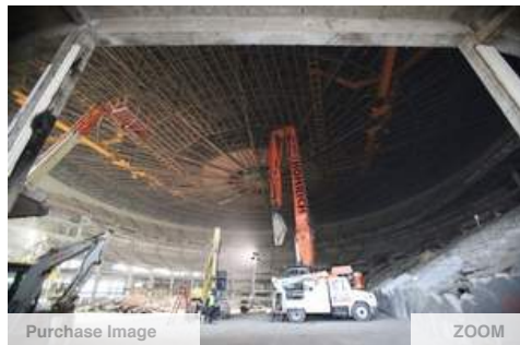
Interior demolition is under way at Cobo Arena as part of remaking it as a dual-level exhibition hall and ballroom. / PATRICIA BECK/Detroit Free Press
